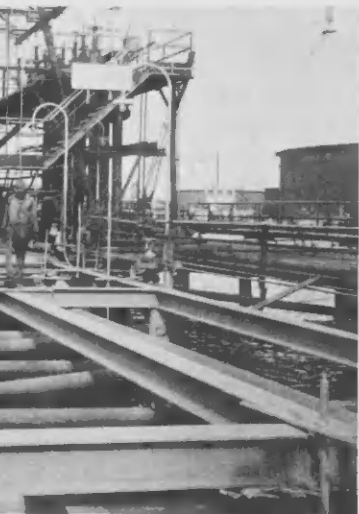
ring system at the West Pier. This work in two shifts. nobo di defensa na West Pier. E trahando den dos warda.
